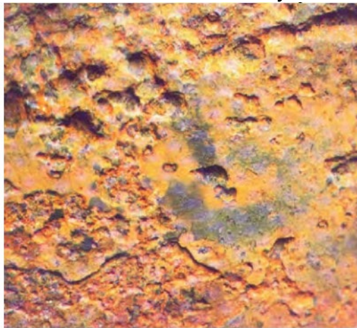
Steel surface affected by MIC
