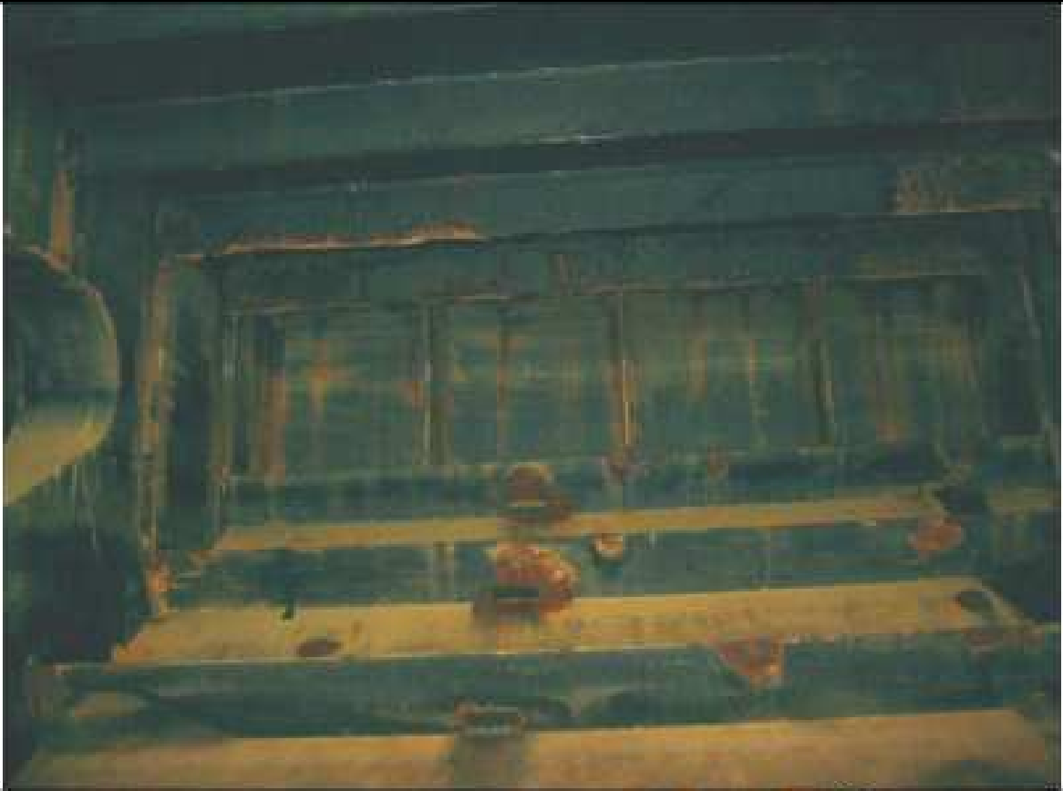
FAIR COATING CONDITION
