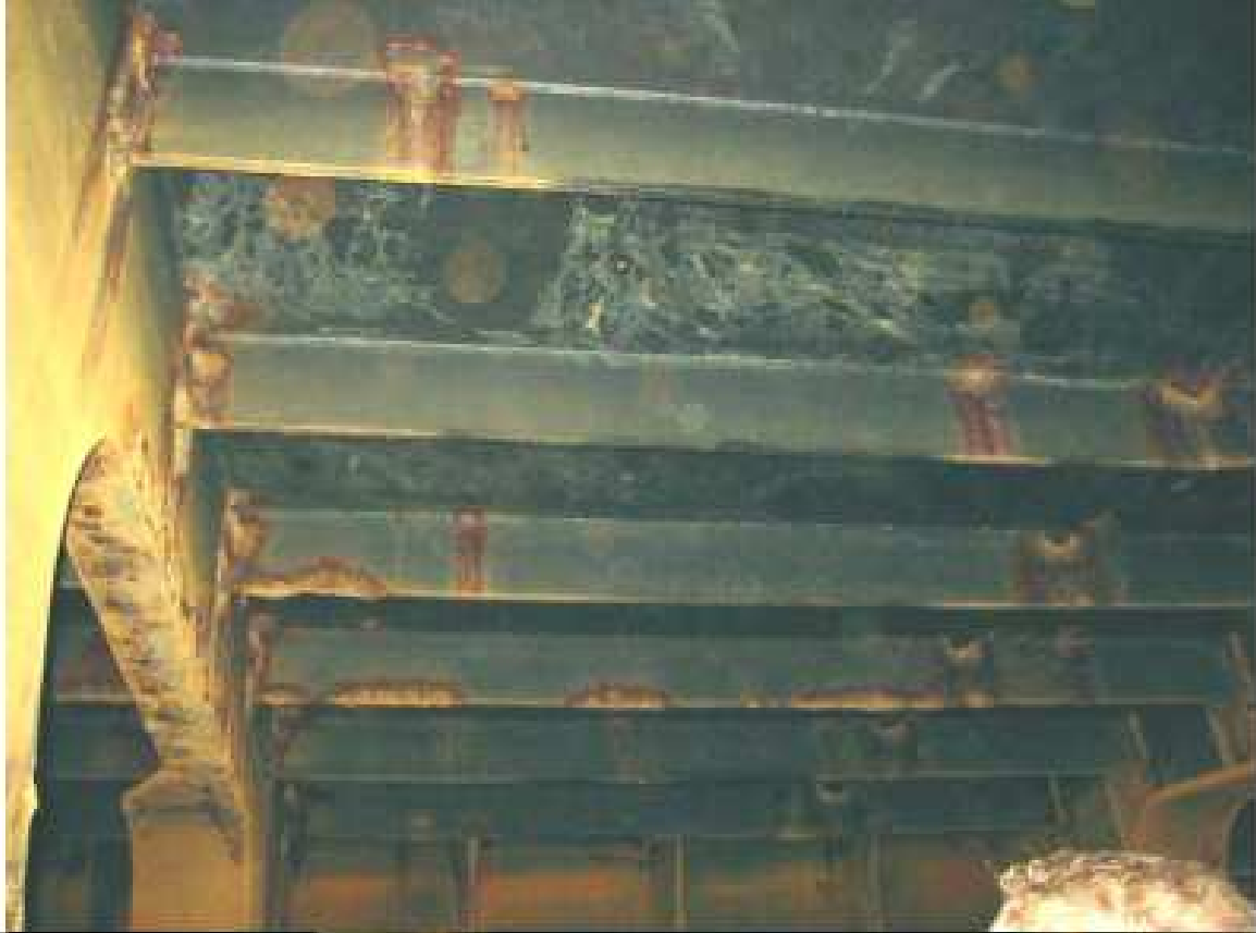
FAIR COATING CONDITION
