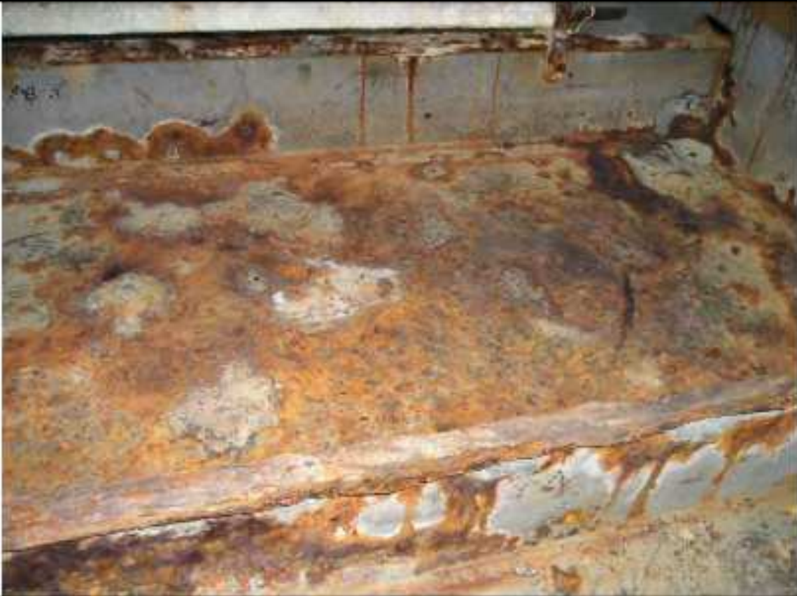
POOR COATING CONDITION
