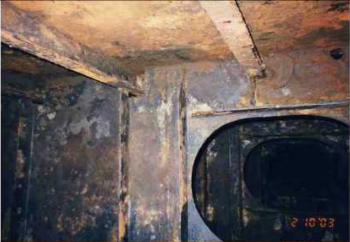
POOR COATING CONDITION
