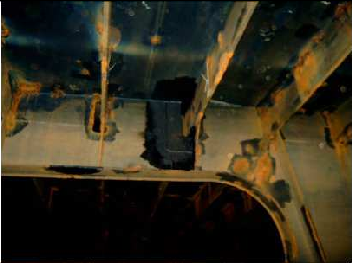
FAIR COATING CONDITION
