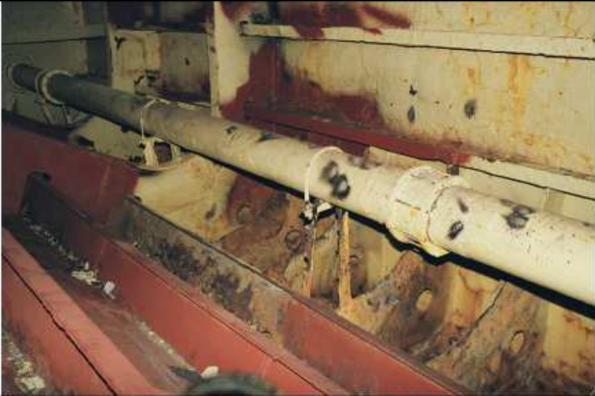
POOR COATING CONDITION
