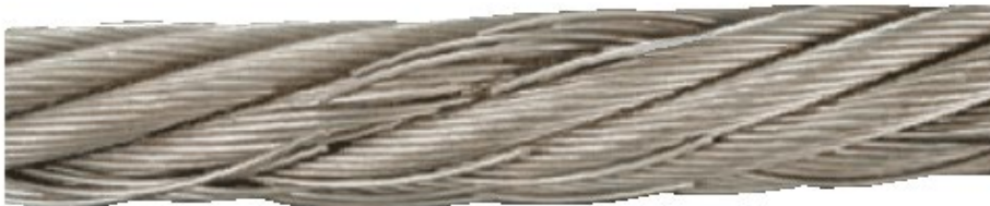
Fig. 3. Wire breaks in one strand, associated with slight wear in a lang's lay rope – further operation is acceptable if this condition represents the worst condition (fractured wires shall be cut out so that the end is at the strand gusset; this prevents further abrasion of the adjacent wires).
